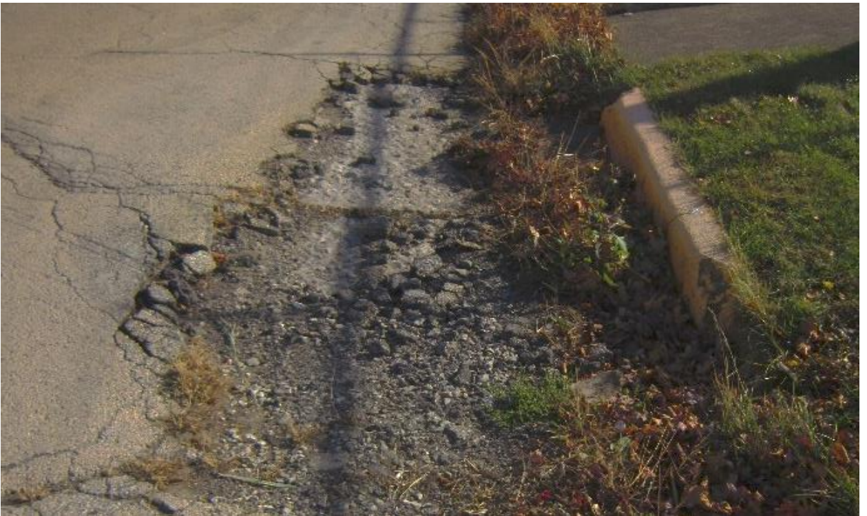
Examples of deterioration throughout the Project Area
