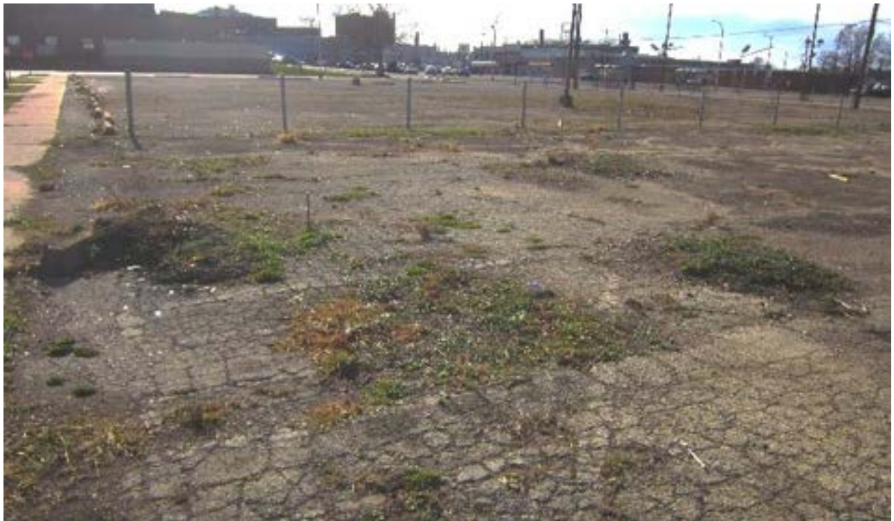
Examples of deterioration throughout the Project Area
