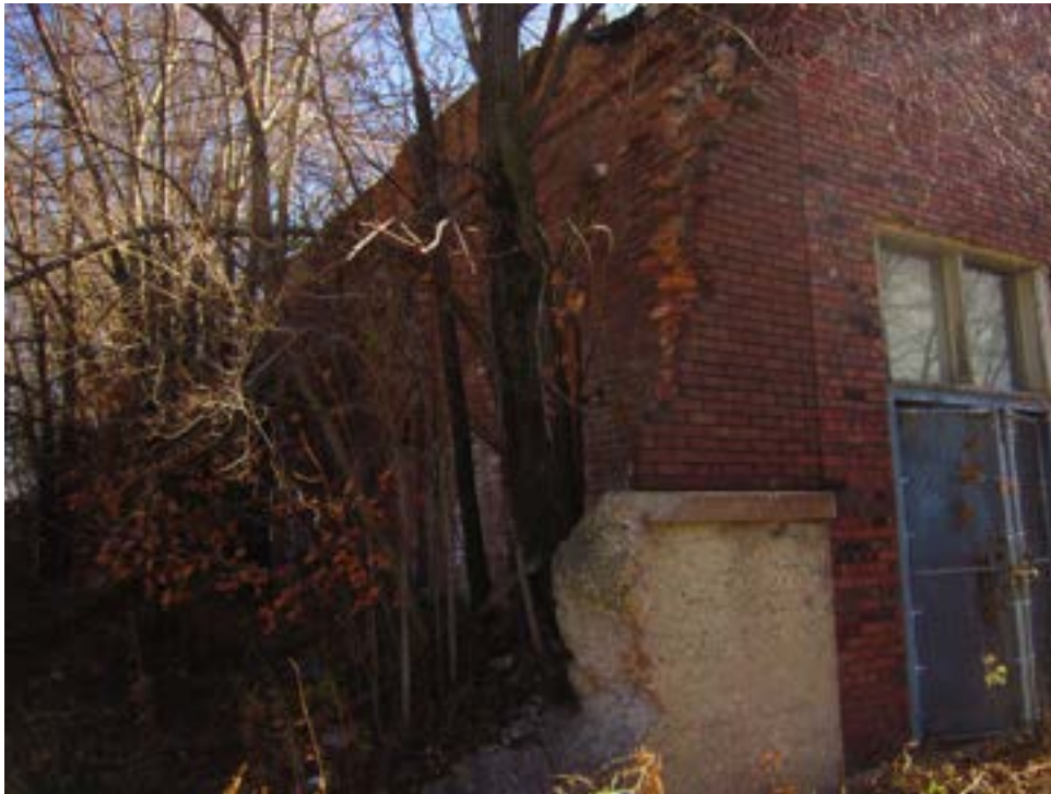
Example of dilapidation in the Project Area
