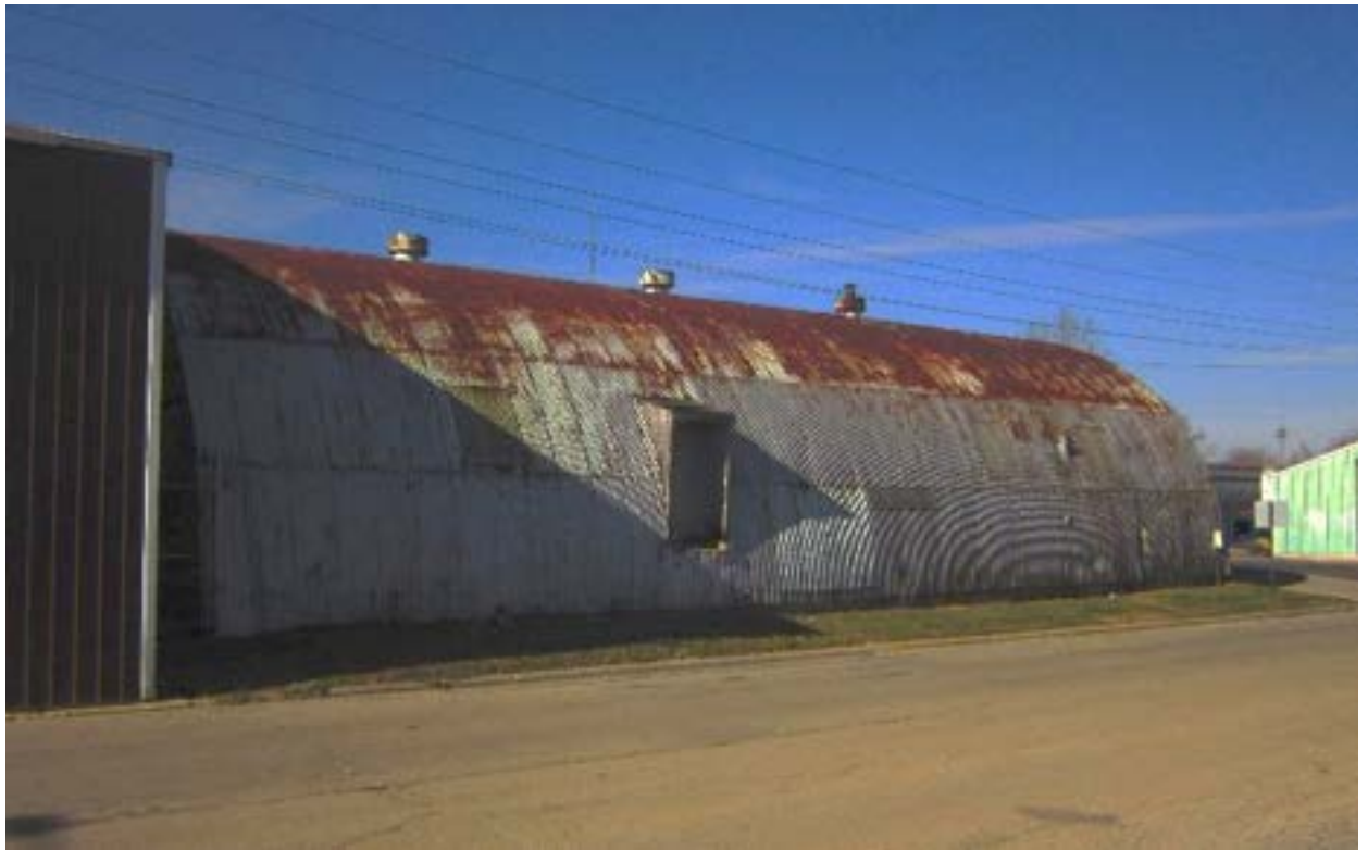
Examples of deterioration throughout the Project Area
