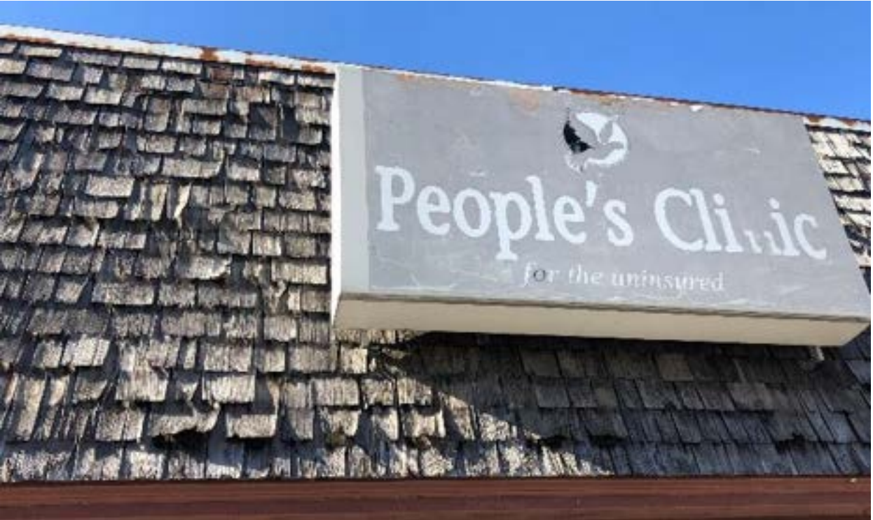
Examples of deterioration throughout the Project Area
